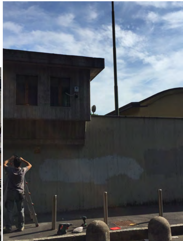
(b) Sensor placement in the facade
