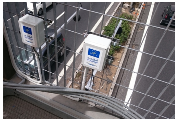
(b) Example of the sensor in its location in the suburban area of Rome (picture property of ANAS S.p.A.).
