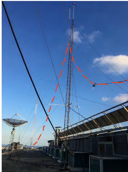
Figure 3.4: Transmitting antenna in Barcelona. Inverted vee antenna made of a flat copper, tunned at 5.4MHz and located in La Salle's Campus. 7
